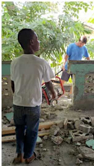
Mr. Massebeau (back) oversees the demolition process in prep for a new missionary home.
