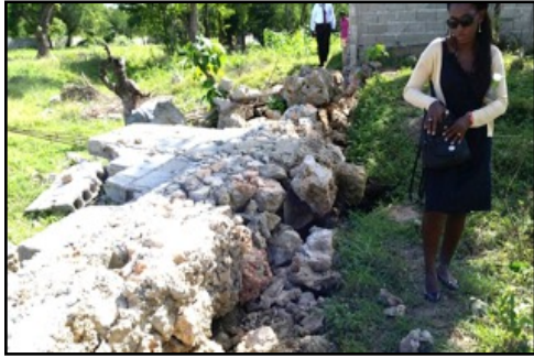
Alexis surveys flood damage to new perimeter wall
